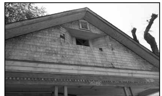
A surprise found under concrete siding.
