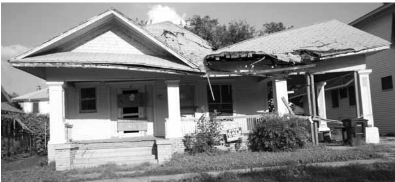
1405 Fairmount Ave. prior to being saved by the Fairmount Neighborhood Association. Once slated for demolition, the home was purchased by Brian and Sheila Portwood and will be open during Home Tour weekend, May 7-8, from noon-6 p.m., as an example of a home undergoing restoration.
