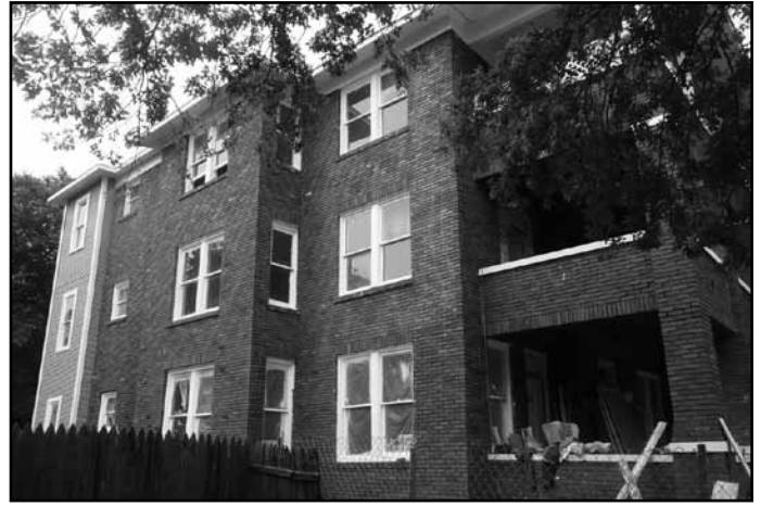
dows. Exterior brick falling off the sides was removed, cleaned and replaced, plus an additional 2,700 matching bricks were found to replace those missing and broken. Thank you Alyssa Banta!
