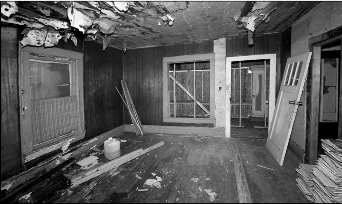
Above: Deterioration after years of neglect will soon be reversed once renovations are complete at 1405 Fairmount. Below: A hall bathroom holds a small clawfoot tub which will remain in the house.
