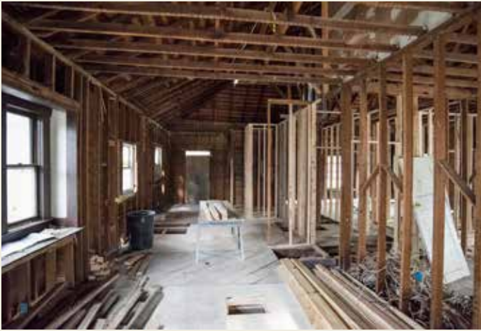
2233 College Ave. undergoes renovation work to convert a duplex single family home back to its original purpose. The bungalow is a part of the Fairmount home tour as a work in progress.
