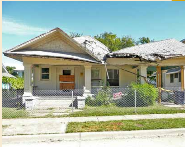
Purchased by the Fairmount Neighborhood Association, 1405 Fairmount Ave. was stabilized and sold for renovation. The house has been completed and the Portwoods are moving in.
