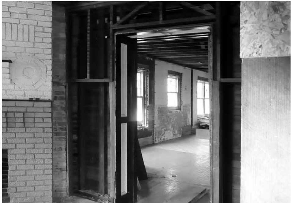
Interior of 1228 S. Adams in 2009. The building has since been rehabilitated while retaining many original features which have either been left intact or reused in other areas.
