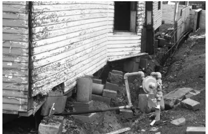
1824 S. Adams with loose blocks, pavers and bricks strewn around the house following a collapsed foundation on Jan. 9.
