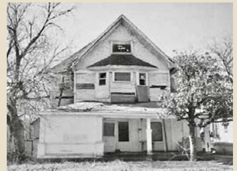
This crumbling house was burned and rotting away, used also as a meth lab. It was scheduled for demolition just hours before it was rescued. Find out what happened to it since on this year's tour!
